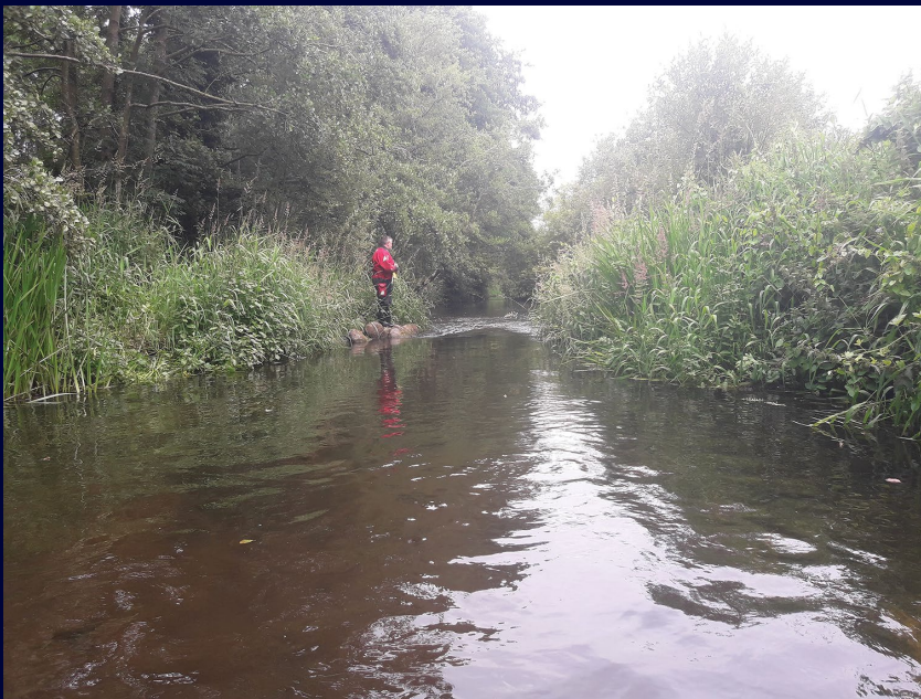
Looking downstream at paired deflectors. This pair of deflectors narrows the flow and speeds it up, introducing diversity.
