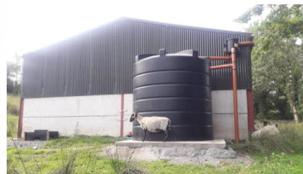
Rainwater harvesting installed at Blacklion Co Cavan
