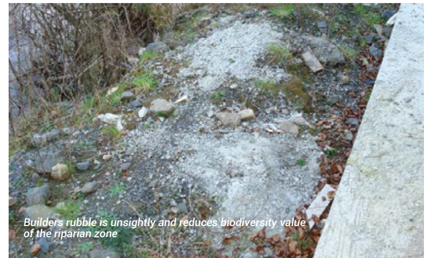
To accommodate this development the adjacent land has been raised too close to the river. This recently built retaining wall almost entirely eliminates the riparian zone and eliminates anglers access. The height of this wall has also introduced another hazard to the area, arguably more dangerous than the river itself to children and local residents.
