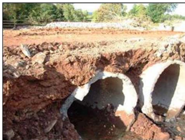
Temporary crossing structure. Impassable for aquatic life and emitting silt to waters as construction equipment traverses the crossing. Unacceptable practice.
