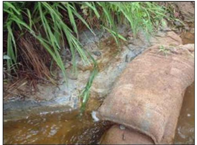
Grout loss to waters is normally stopped by placing dry cement over the leak, with sand bags on top to restrict grout flow until the leak solidifies. (This photograph was taken after water flow was re-established following solidification of the grout.)
