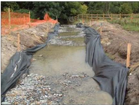
Terram lined (to prevent erosion) silt control pond outlet channel showing gravel acting as filter medium for silt removal.
