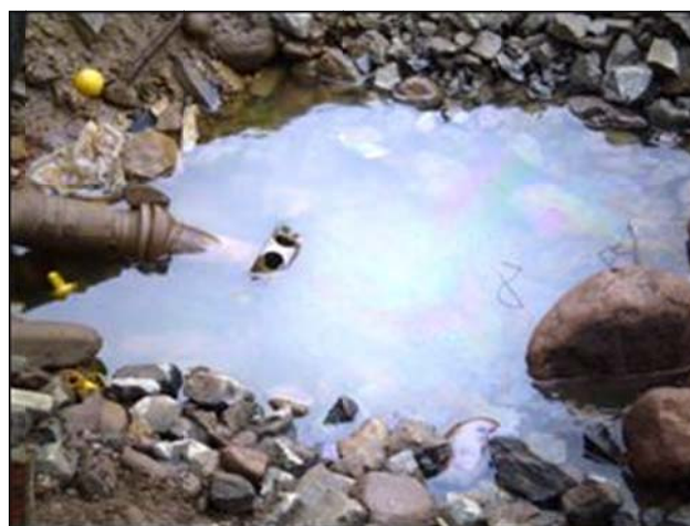
It is a serious offence to discharge deleterious matter such as oil contaminated residues to waters.
