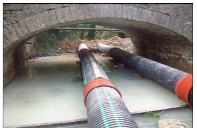
Repairs to a single arch bridge and scour slab with stream flow piped from upstream to downstream (foreground) during both grouting and slab repair.
