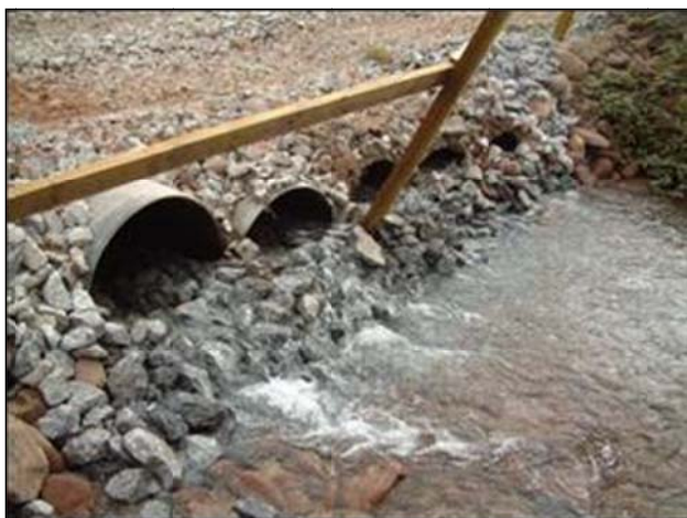
Temporary crossing impassable to fish life.
