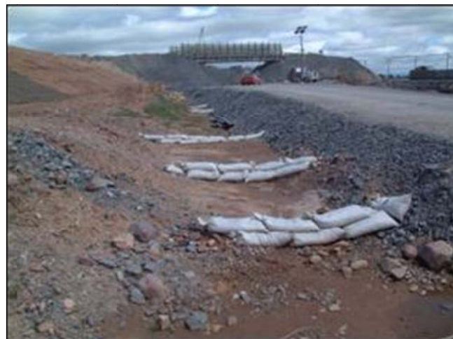
Silt discharge minimisation by providing retention areas to reduce discharge velocity and allow settlement during rainfall events.
