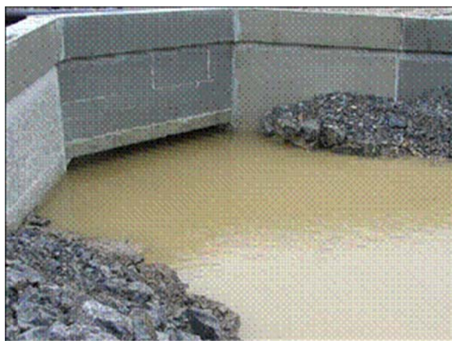
Is the culvert adequately sized?
