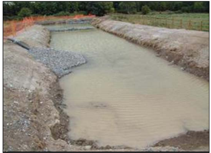
Silt control pond. Note hose conveying pumped silt laden waters with its outlet positioned within the gravel mound thus ensuring no disturbance of pond contents.
