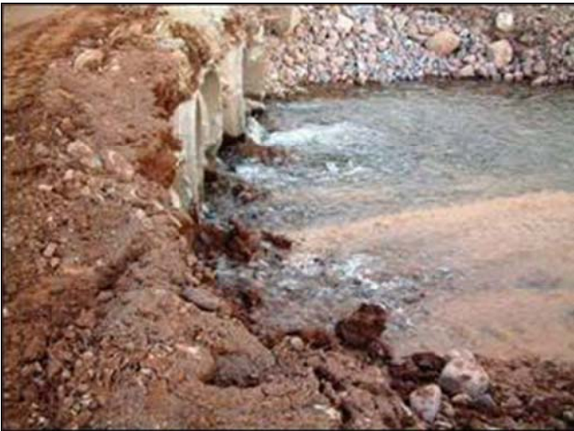
The inevitable result from the crossing shown above. Continuous silt discharges. Unacceptable practice.
