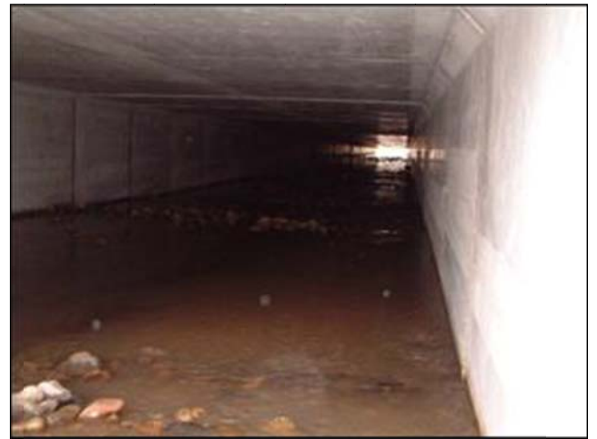
Excessively long culvert resulting in habitat loss and reduced productivity due to inadequate light penetration.
