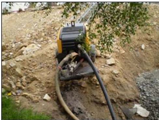
Drip tray is undersized, dangerously positioned and leaking oil. Unacceptable practice.
