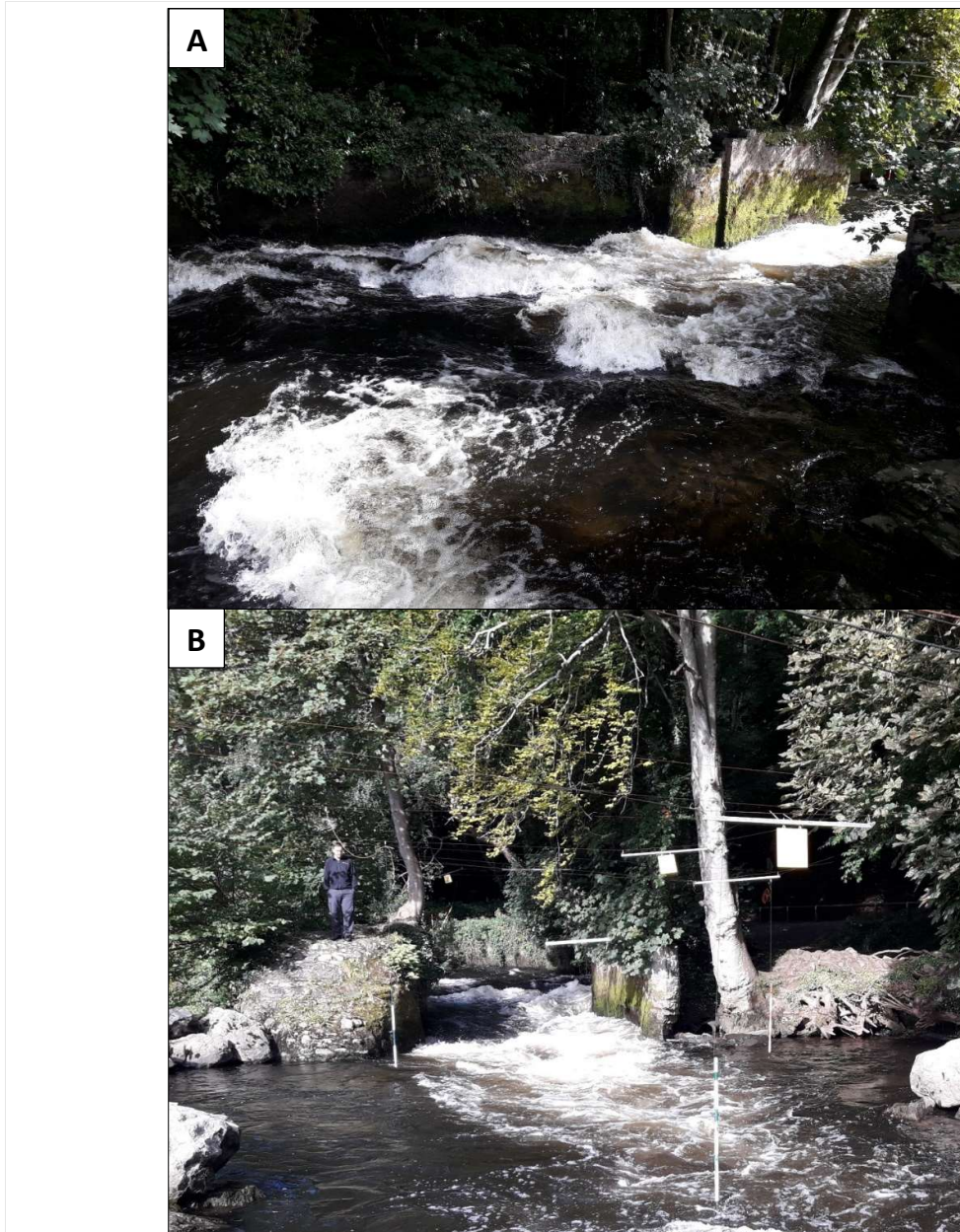
Figure 38. Breached sluice from (A) upstream and (B) downstream (TS1).
