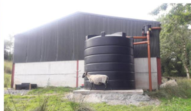
Rainwater harvesting installed at Blacklion Co Cavan
